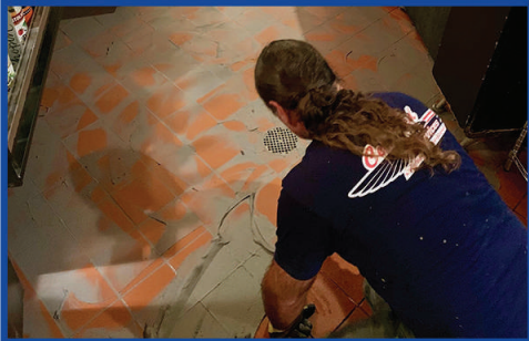
Tile & Grout Repair
